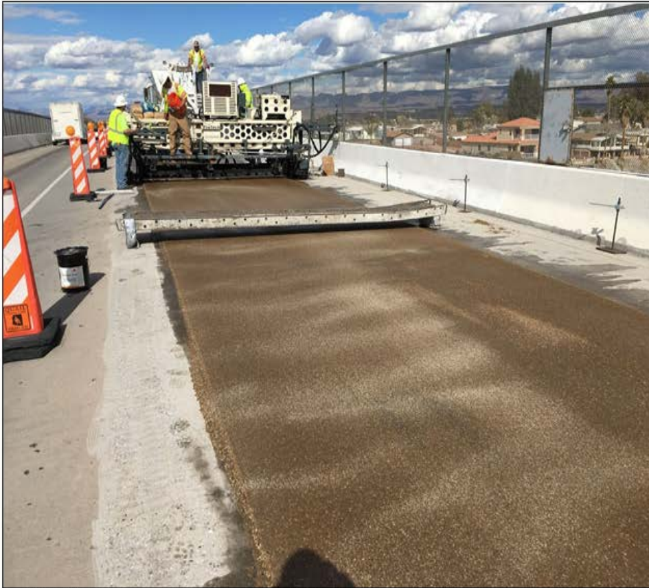
Picture: Paving is now complete on the SR 95 Needles Bridge deck overlay project.
